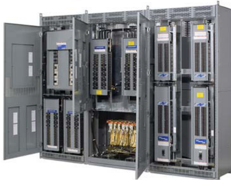
Integrated Power Center 2
