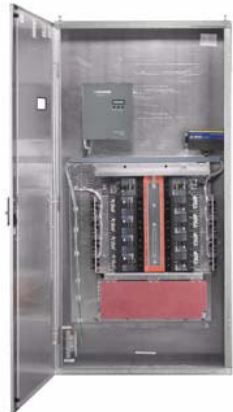
Submetering Integrated Power Center
