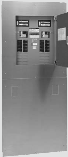
Duplex Isolation Power Panel, see page 15-3
