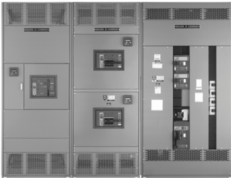
QED-2 Switchboard (Class 2742)
