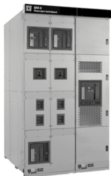
QED-6 Switchboard (Class 2746)
