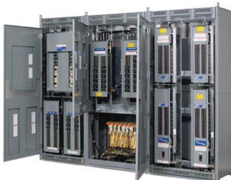
Integrated Power Center 2
