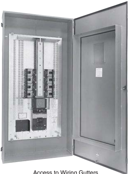
Access to Wiring Gutters
