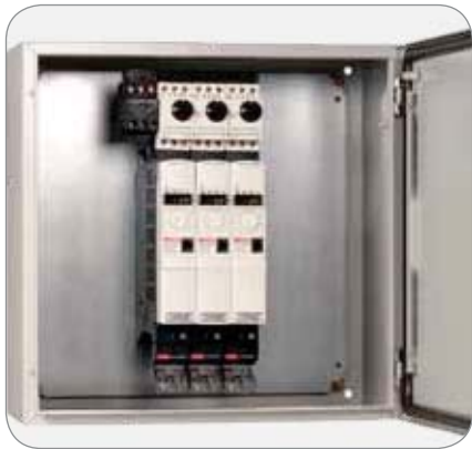
Power supply and protection for several drives by means of a busbar and GV self protected disconnect.
